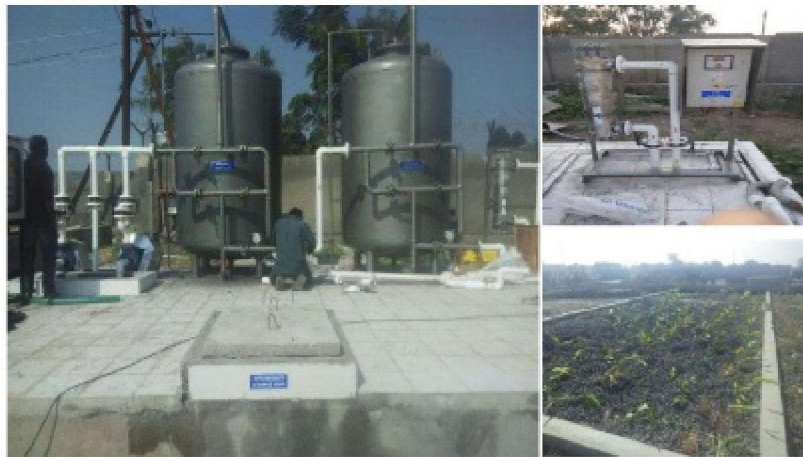
Sara Builders & Developers Pvt. Ltd. - 500 CMD STP
